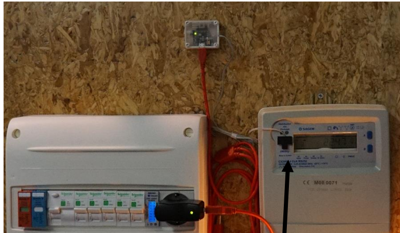
Sensor applied in the energy Meter
